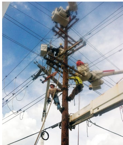
IBEW Local 113 and traveling journeyman linemen work to restore electrical power after a storm.
